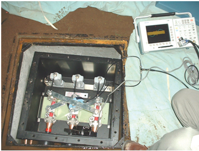
Figure 6. A PD sensor was placed at the link that short-circuits the cross bond
