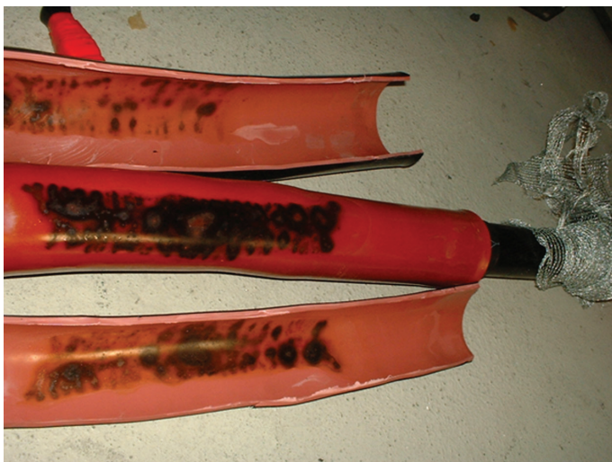
Figure 12. PD burn marks between two layers of sleeves of a joint
