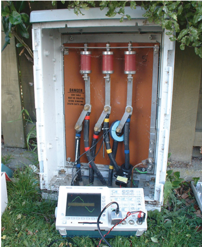
Figure 8. PD sensor was clamped on the cross-bond earth
